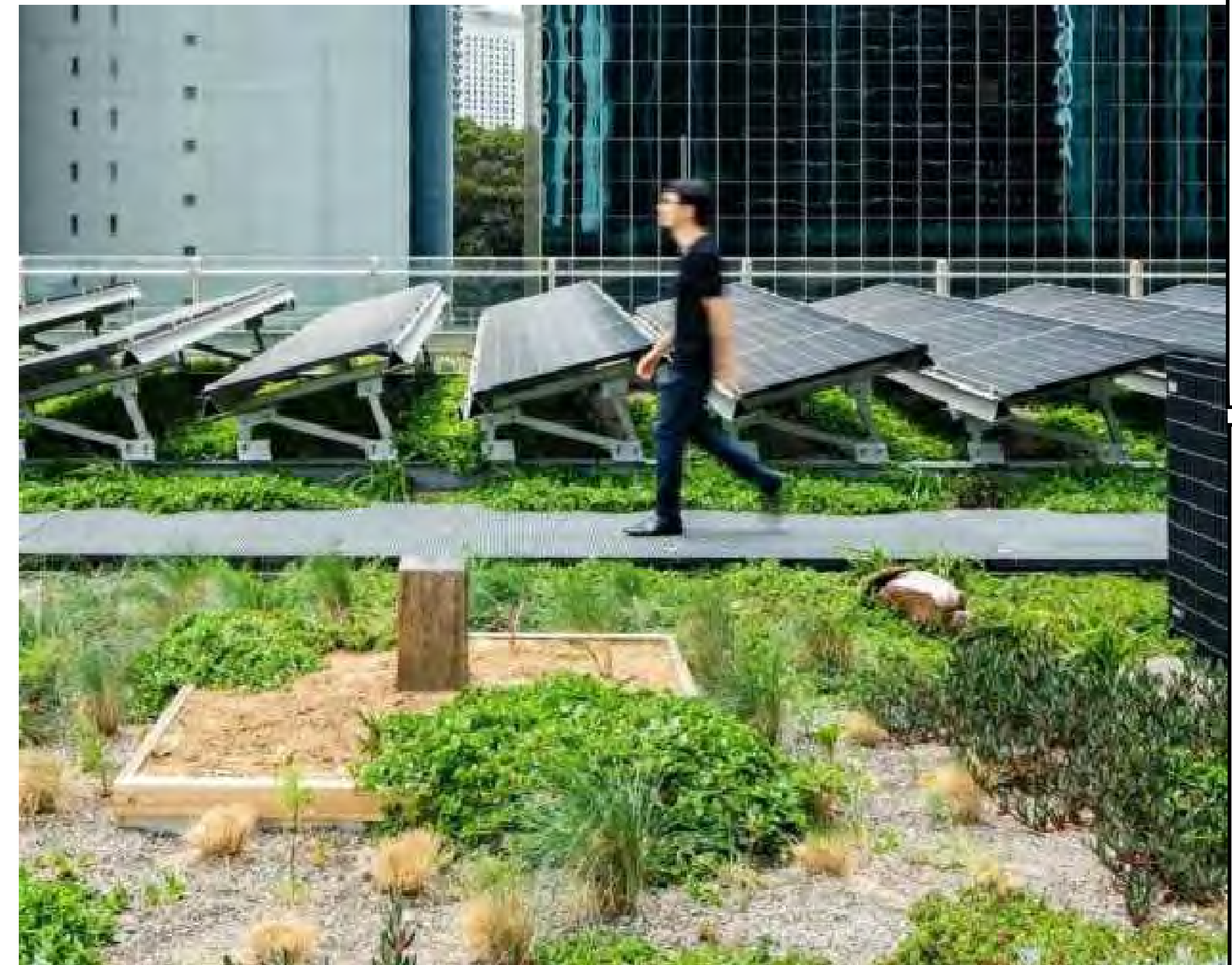
GREEN ROOF & SOLAR PANELS
